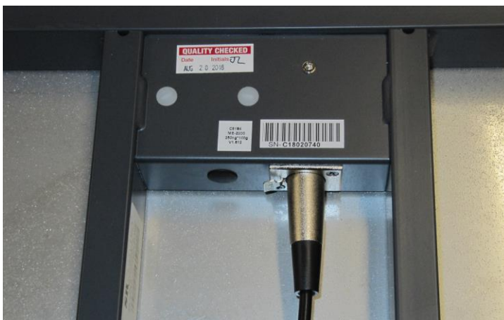
Figure 2: Cable Connection to Platform
